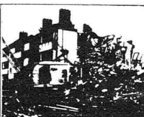
Since 1983 over 6,000 unsatisfactory council properties have been or are being demolished in Liverpool.
