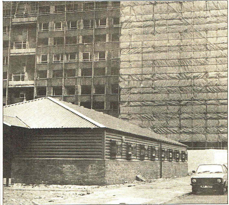
New neighbourhood housing office in front of the infamous Piggeries blocks being demolished.
