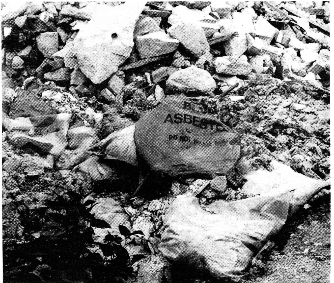
Lethal blue asbestos lying scattered on a building site in Lambeth, South London
