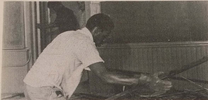
Marcus Garvey, custodian cautiously steps through fallen ceiling.
